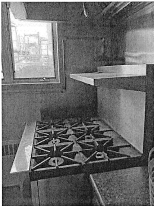
Stove and exhaust hood
