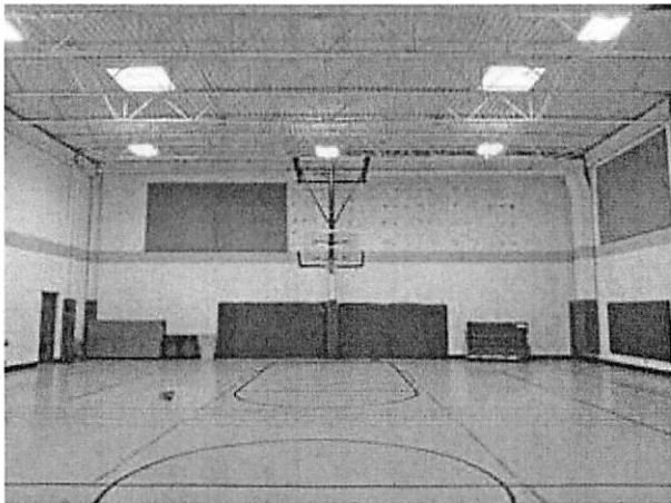
Missing acoustical padding at upper walls
