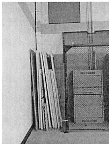
Makeshift storage between electrical cage and wall
