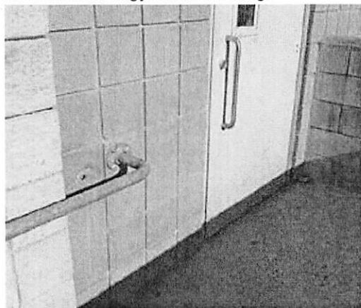
Holes in masonry from handrail support.
