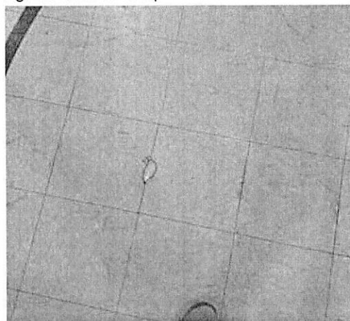
Damaged floor tiles
