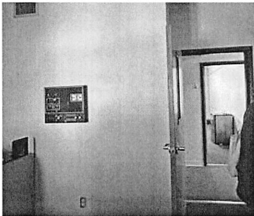
Existing wall-mounted answering machine
