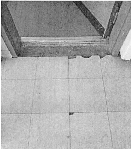
Damaged floor tiles at entry to egress stair
