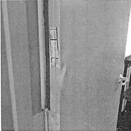
Door to kitchen is damaged
