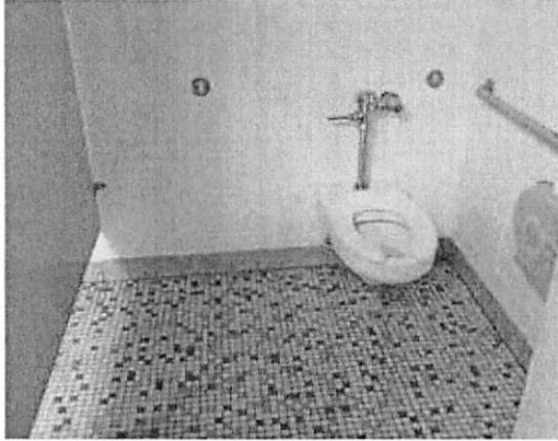
Accessible stall missing rear grab bar. Height of toilet seat is 15" AFF.
