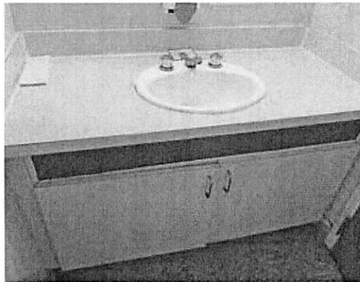
Men's toilet: Sink cabinet missing panel
