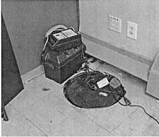
Exposed sump pump
